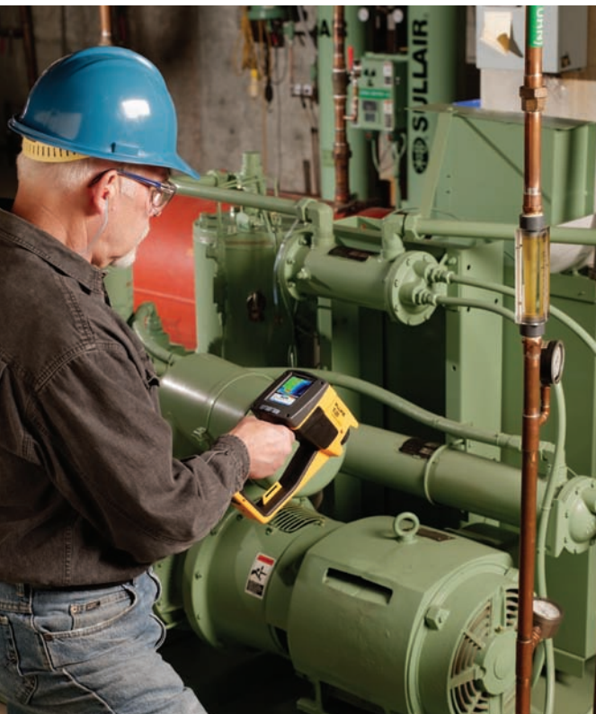
Figure 1. Thermal imagers offer a quick way to inspect equipment for abnormally hot-spots, and piping for abnormally cool spots.
