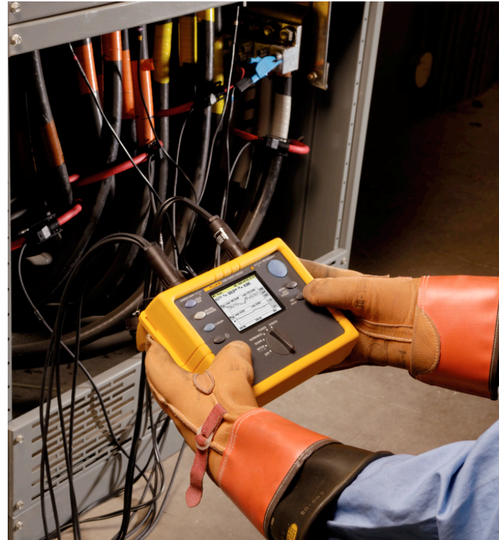
A three-phase power logger can measure demand over time, which can help identify areas where companies can cut energy costs.
