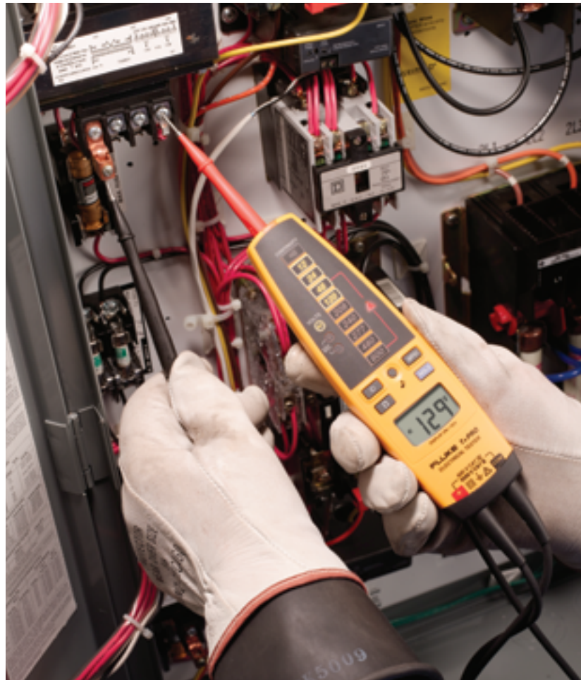
Testing control voltage on a 480 V panel controlling two small chiller pumps.
